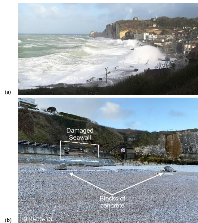
Figure A1. Seawall damages in Etretat on 12 Mar 2019 after high-energy conditions (a); damage to Etretat's seawall after a storm in early 2020 (b).
