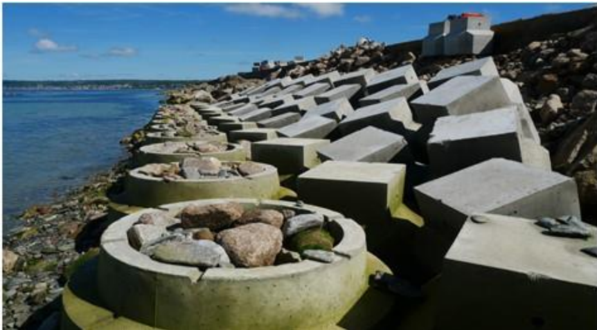
Figure 4 - ACCROBERM™ II toe blocks filled with rocks (at the bottom of the repair solution) interlocked with Double-Cube blocks placed on the slope
